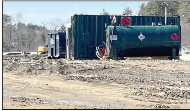
Landry French will serve as the General Contractor for the new Windham Raymond Middle School at its location on Windham Center Road. The site is currently being prepared, and materials are being delivered. Construction is expected to start soon and the school could by August 2027. PHOTO BY ED PIERCE
