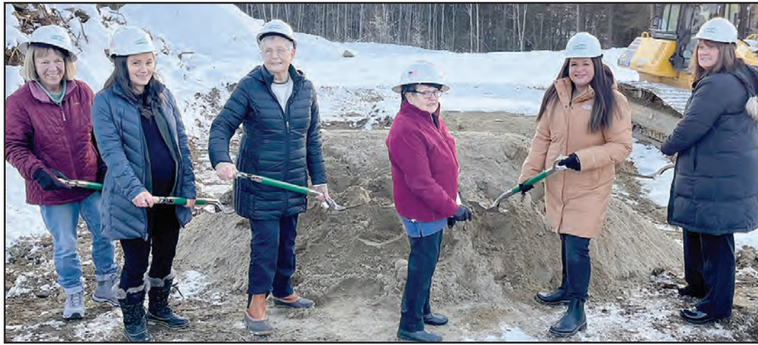
Windham/Raymond School Age Child Care held a groundbreaking Tuesday for its new 'Space to Thrive' facility on Pope Road in Windham. From left are Pam Whynot, Board member; Hannah Marshall, Executive Director; Donna Cobb, Board President; Jeanette Lamb, Board member; Julia Champagne, Project Manager; and Sherri Evans, Board member. SUBMITTED PHOTO
