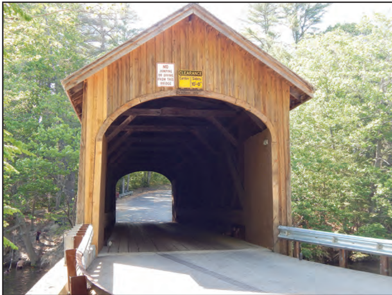
Crews have started working on repairing Babb's Bridge in Windham after a truck exceeding the established weight limit crashed through the bridge floor into the Presumpscot River last August. The repair project is expected to take about six weeks to complete before the wooden covered bridge can be reopened. PHOTO BY ED PIERCE
